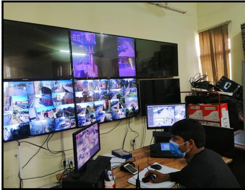
Control room operator observing/checking all security measures with CCTV cameras/Walkie talkie/ Emergency 15 android application
